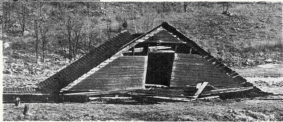
COLLAPSE: Down went the icehouse! Nobody was inside at the time. David Milner
